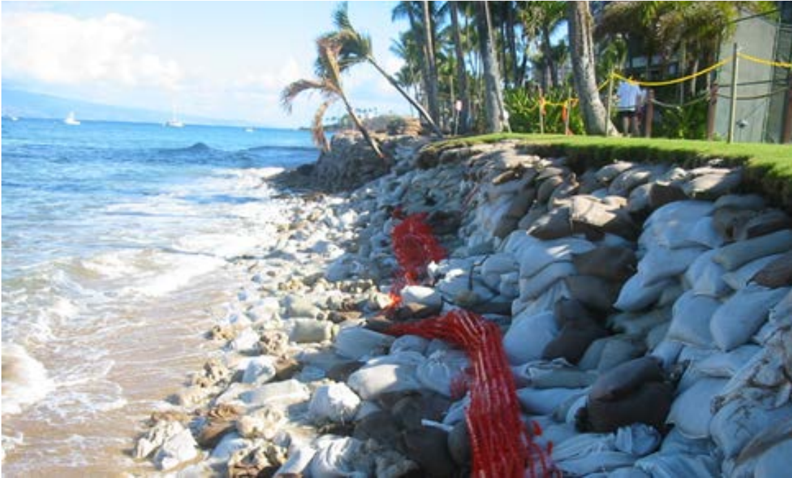
Sandbags protecting buildings on an eroding shoreline. Image courtesy C. Fletcher
